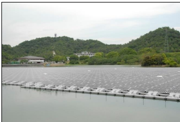
2.3MW plant in Kasai City
